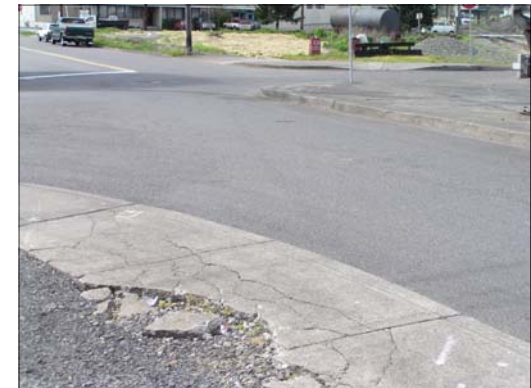
Broken cement slowly erodes the amount of walkable space on the sidewalk.
