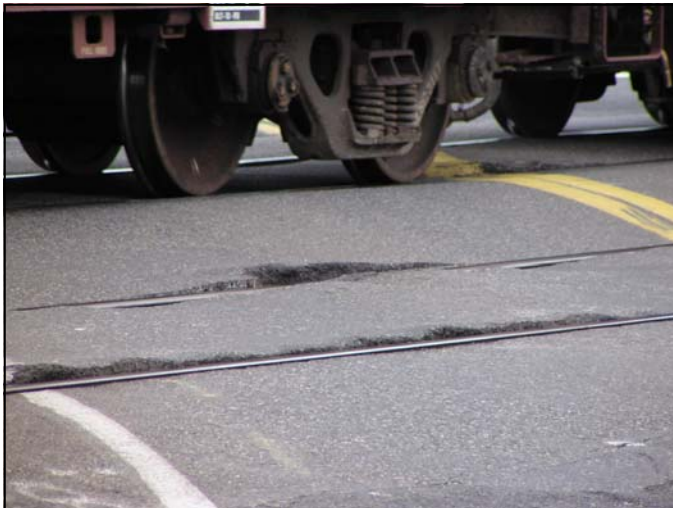
Poorly maintained railroad track with large gaps and uneven pavement
