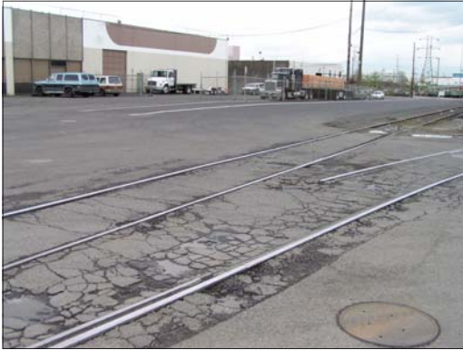
Broken asphalt and angled railroad tracks pose as a hazard for bicyclists.
