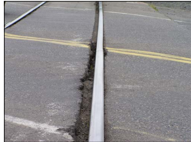
An undesirable railroad crossing condition for bicyclists
