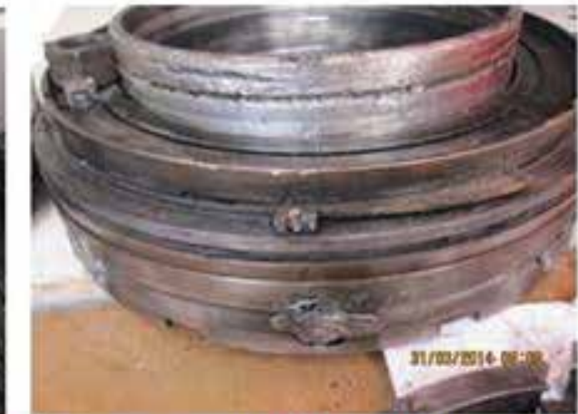
3 Primary seal with plug vent & supply ports with melted part
