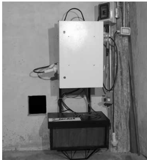
Figure 94. The batteries were installed in a movable device; hence, it can become an emergency power plant if needed. Photo by Claudia Garduño.
