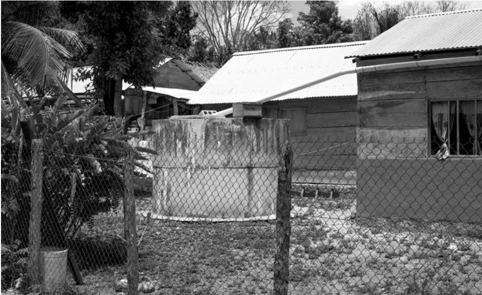
Figure 50. The water harvesting system that most houses in El 20 have, with the 12000 litres water tank, and the PVC tube connected to the rooftop. Photo by Jan Ahlstedt.
