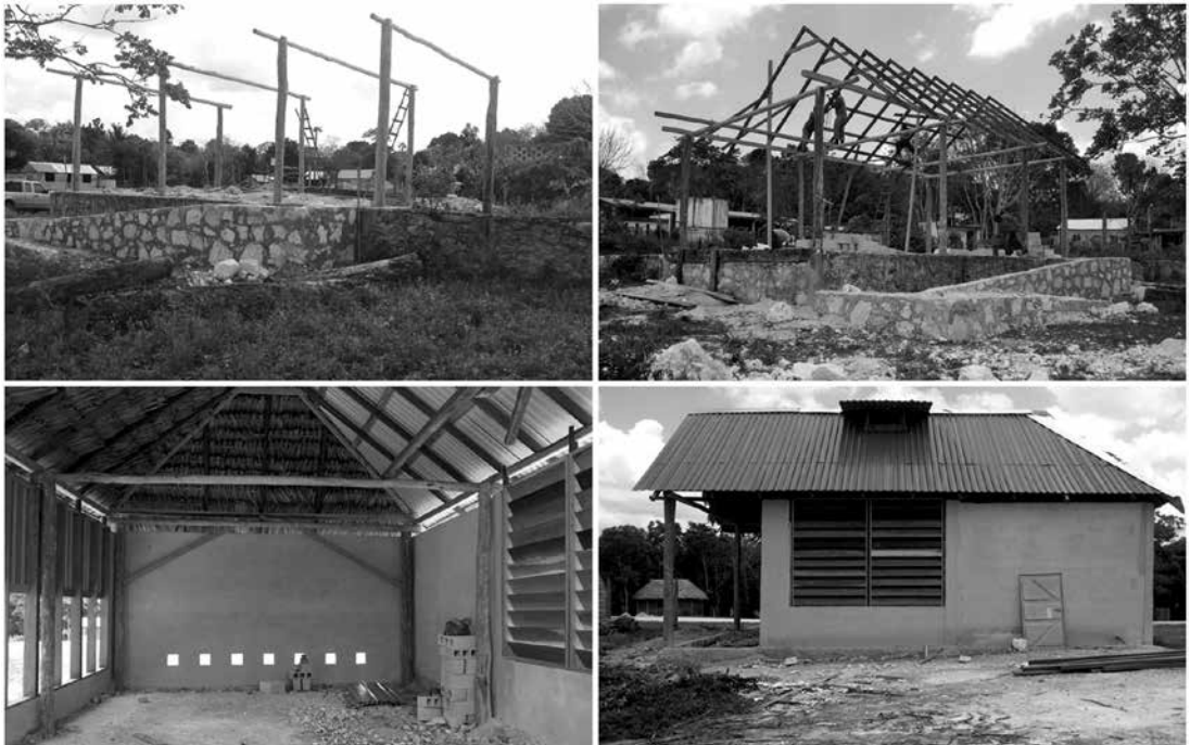
Figure 92. Some pictures sent by Miriam Cabuich at different stages of the construction. Published in Garduño 2015 (121).
