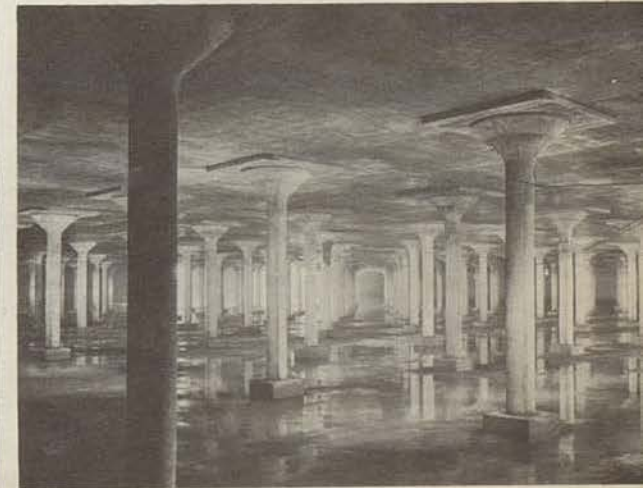
To ensure an adequate supply of water, the Windsor Utilities Commission maintains underground storage facilities having a capacity of 11 million gallons.
