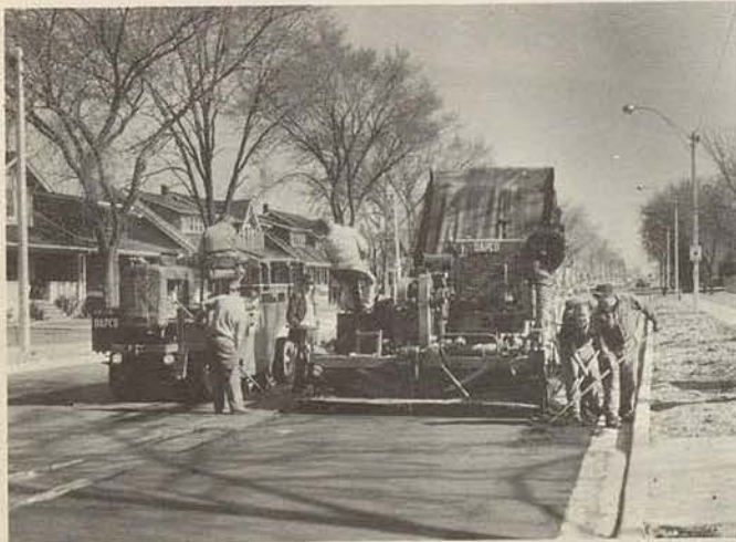
In maintaining street surfaces, the Public Works Department operates an Asphalt Plant producing 20,000 tons of paving material a year.
