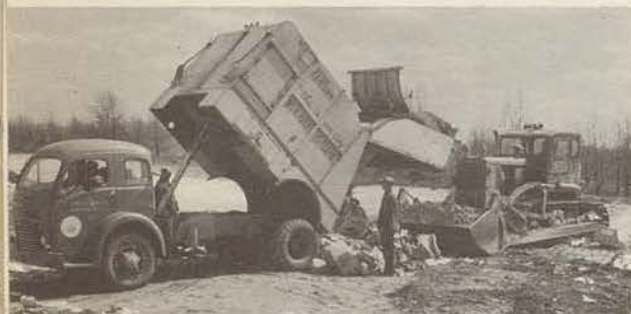
The modern sanitary land fill method of garbage disposal has now replaced incineration and unsightly dumping. The City's 80-acre landfill site will ultimately be developed as a municipal golf course.
