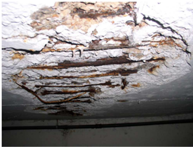
Figure 1.1 Deteriorated slab (Hoffman Architects,2014)
