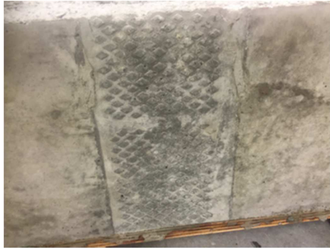
Figure 3.11 Irregular pattern of concrete surface after removal of plastic strip
