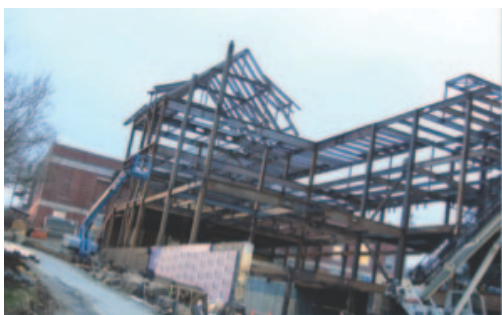
3/24: Progress on Hamilton Smith Hall was detailed in the March 24 issue, as computer-generated plans for the renovation were also released. The projected time of completion for the project is fall 2017.
