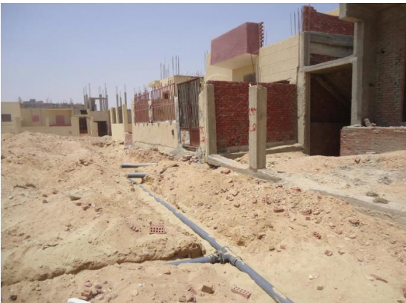
Figure 4: Infrastructure construction in 6th of October City—de facto this often happens long after the allocation of plots and construction of housing units.
