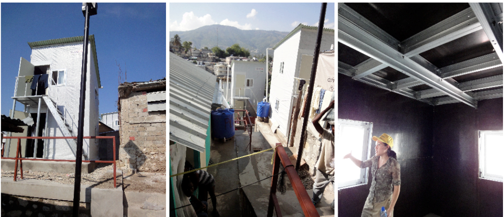
Figure 2: The two-story houses were designed to last for two or three years. Each building is able to host two families.
