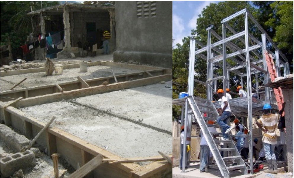
Figure 1: From left to right, stages of the construction: the concrete foundation is resistant to seismic and wind stress, neighbors erect the steel frames which constitute the structure, which is then covered with plastic sheeting on the exterior and plywood in the interior. ▸
