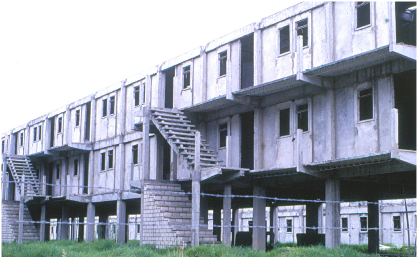
Figure 11 a through b: Ciudad Bachué, Bogotá Colombia (Source: UNAL, undated) Above: structural frame to support vertical extensions of up to 5 floors (approx. 1978) Below: structural frame with wall panels (approx. 1979)
