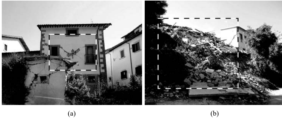
Figure 11 Complete collapse of (a) masonry wall and (b) diagonal cracking due to shear failure (Amatrice)
