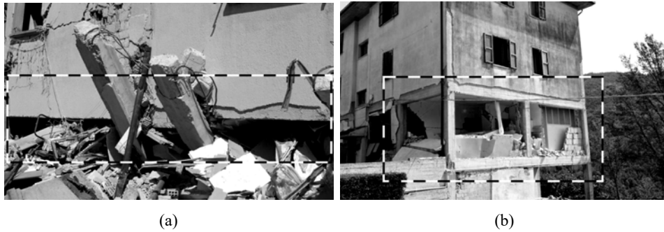
Figure 12 (a) Ejection of the infills (Arquata del Tronto) and (b) soft storey mechanism (Amatrice)
