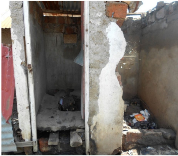
Figure 2 . A dysfunctional pit latrine: it was full and had collapsed.
