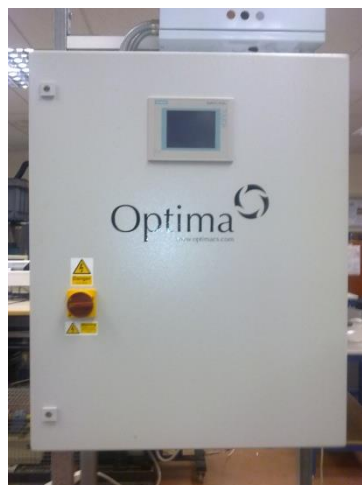
Figure 6-12 Test rig control panel
