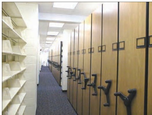
Compact shelving installed on the ground floor of Aloysia, with tracks that carry the enormous weight of more than 11,000 linear feet, over two miles, of books.
