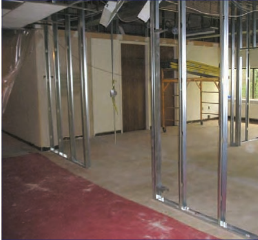
New walls divide the Library reference staff offices in the old Registrar's space
