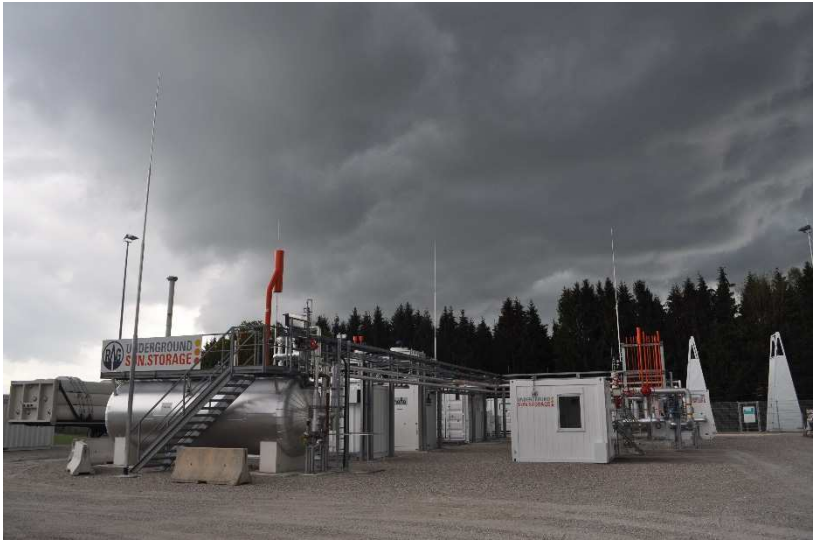
Figure 4 – A geological underground storage site for methane (90%) and hydrogen (10%) mixture at a depleted natural gas reservoir near Pilsbach, Austria Photographed by MUNKÁCSY, B. (2016)
