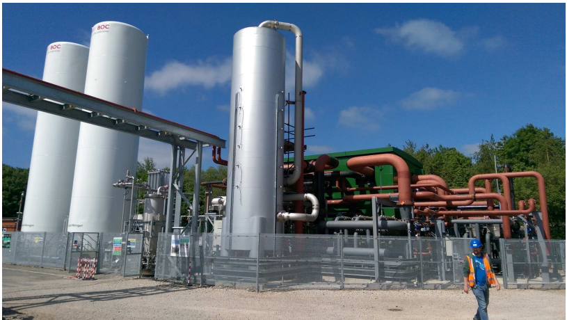
Figure 9 – Pre-commercial demonstration plant
