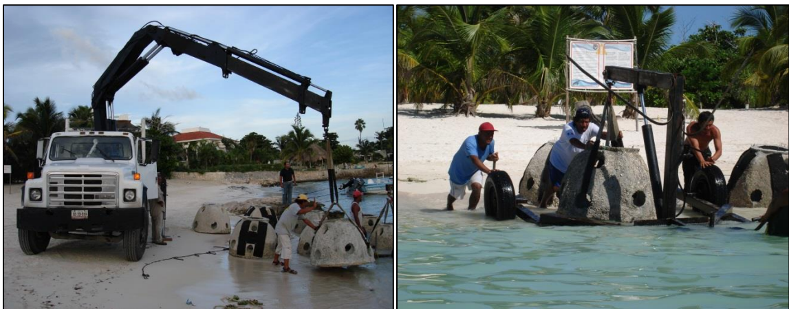
Figure 2.11 Modules being offloaded (left) and moved into the water (right) in Akumal.
