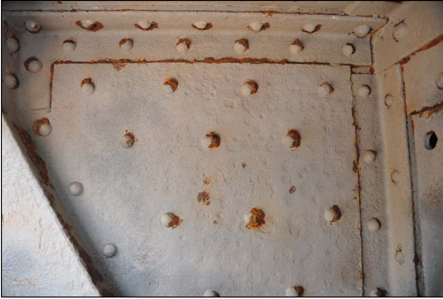
Fig. 5: Pitting corrosion of a steel plate.
