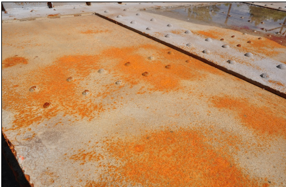
Fig. 4: Deterioration of a steel cover plate.
