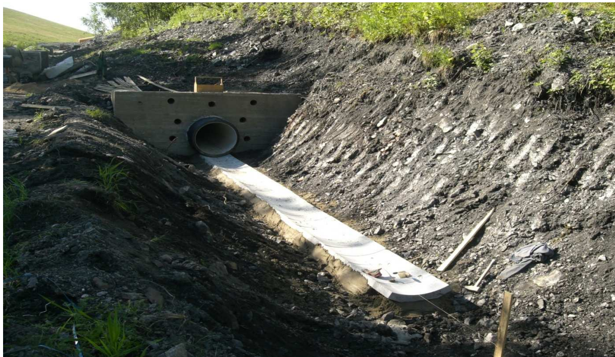
Fig. 4. An example of ground shaping in the Central Heap – ditches and protective bunds [1].
