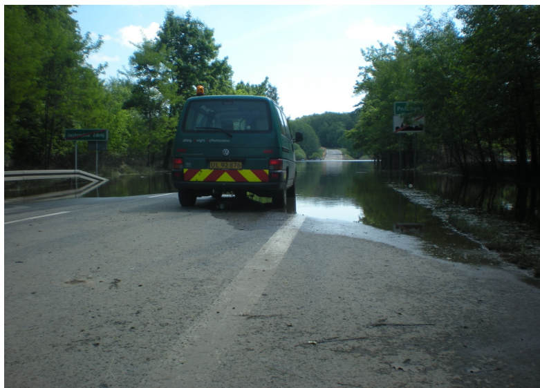
Fig.5: Deluged pavement surface of Voivodeship Road 933 in June 2010
