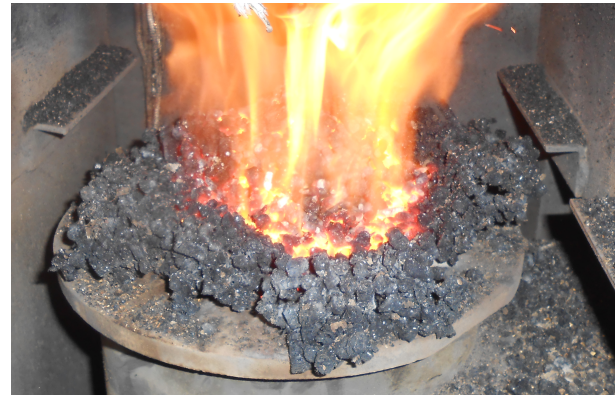
Fig. 5: The combustion chamber of the boiler during alternative pellet combustion.
