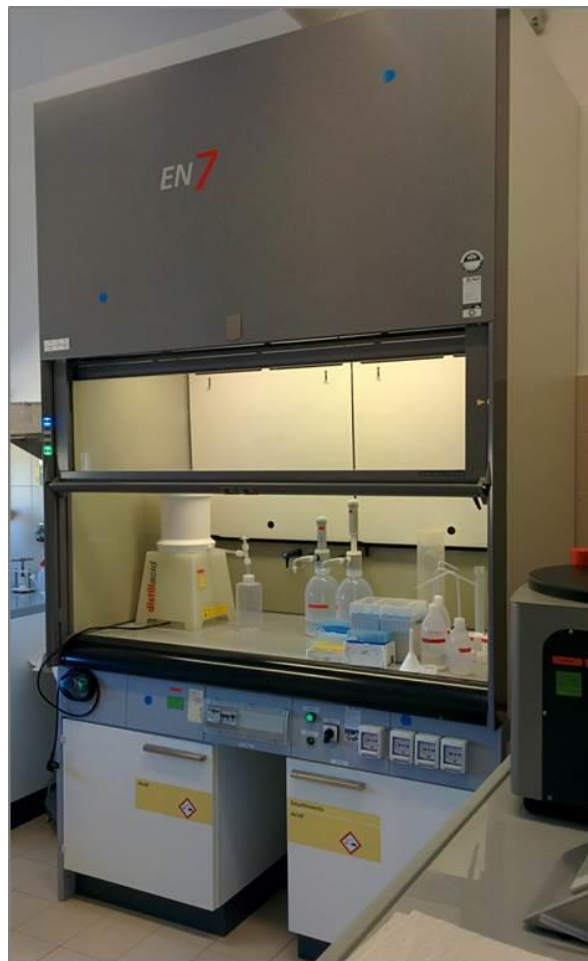
Figure 3.5 Clean Laboratory equipment: fume hood for acid treatment.
