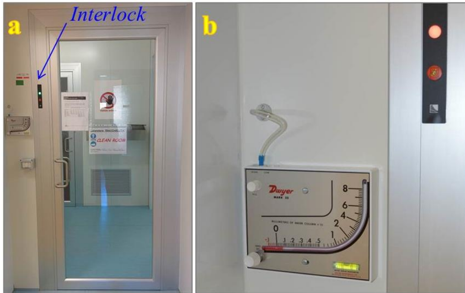
Figure 3.8 The interlock system a) and the pressure control system b) that measures the pressure between the dressing room and outside.
