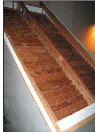
Figure 68: The wood louvers in Roof Module 1 before the corrugated roof was installed.
