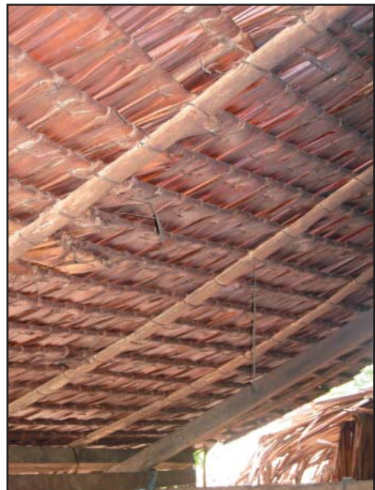
Figure 30: This shows the underside of a palm thatch roof. Since the palm thatching is light in weight, the structure can also be very light weight.
