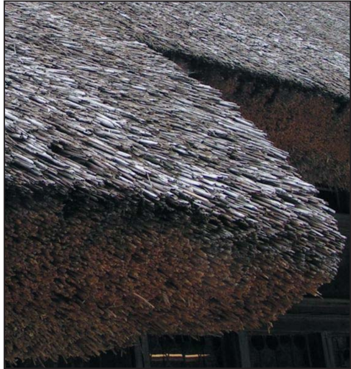
Figure 27: This is the edge or eave of a water reed thatch roof. The thickness of the material and the air pockets in the reeds make this a thermally insulated roof suitable for colder climates.
