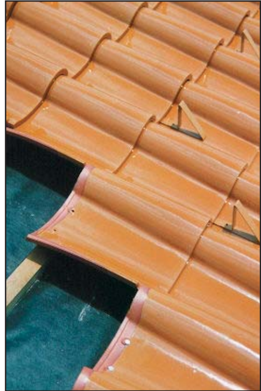
Figure 44: These are glazed “S” clay tiles during installation. The wood mounting strips are visible and the underlayment to prevent any leakage. The brackets on the top of the tiles are snow clips to prevent snow from sliding off the roof . ( http://www.rooftilemanagement.com/Images-Products/Tile/TerraCotta/Large/Glazed_Clay_Tile_3.jpg )
