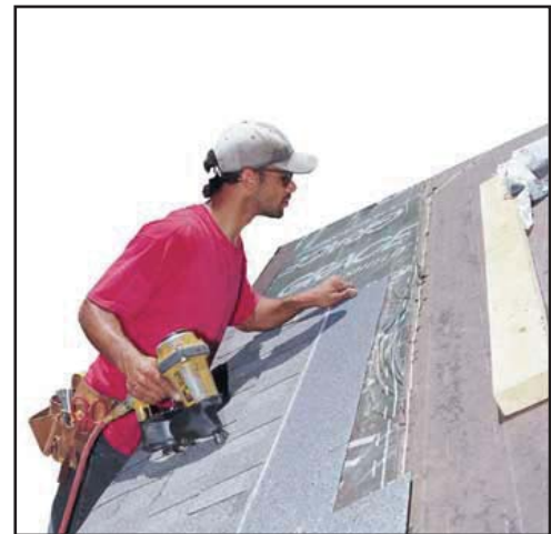
Figure 34: Pneumatic air guns are now being used instead of hammers to install the shingles which cuts the installation time in half.
