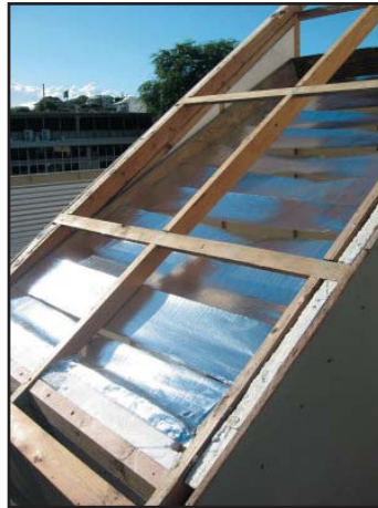
Figure 70: The radiant barrier louvers in Roof Module 2 before the installation of the corrugated roof.
