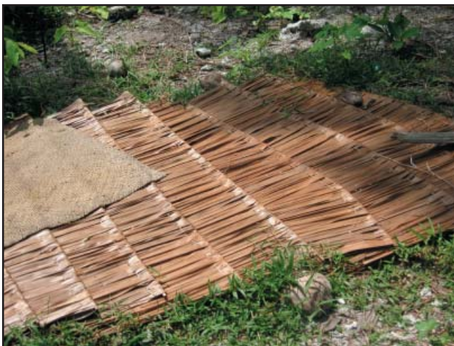
Figure 29: This shows the preassembled thatched palm panels which will be installed on the roof. These panels are easily repaired and replaced.
