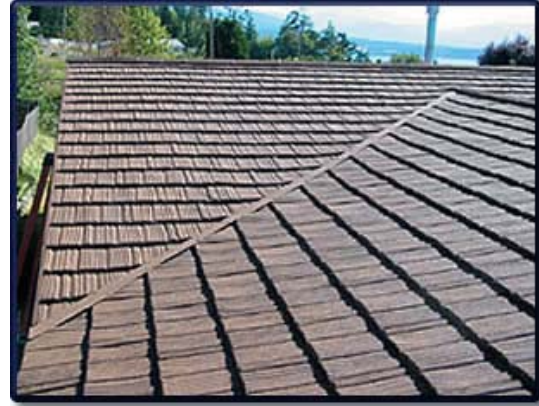
Figure 53: This is a metal roof even though it looks like a shingle or shake style roof. ( http://www.olympicsteelwa.com/images/105_0521_frame )
