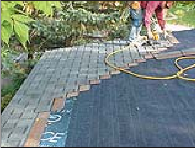
Figure 33: Shingles being applied over asphalt felt underlayment. The shingles are started at the eave and are staggered up the roof to the ridge.
