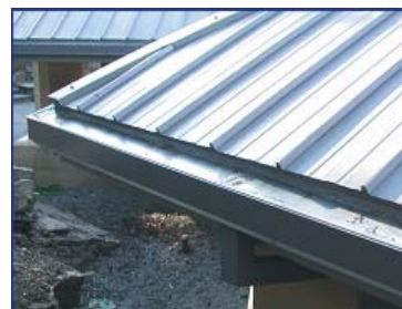
Figure 51: Metal roof are commonly used with water catchment systems, This is due to smooth surface that resists mold, mildew, and fungal growth.
