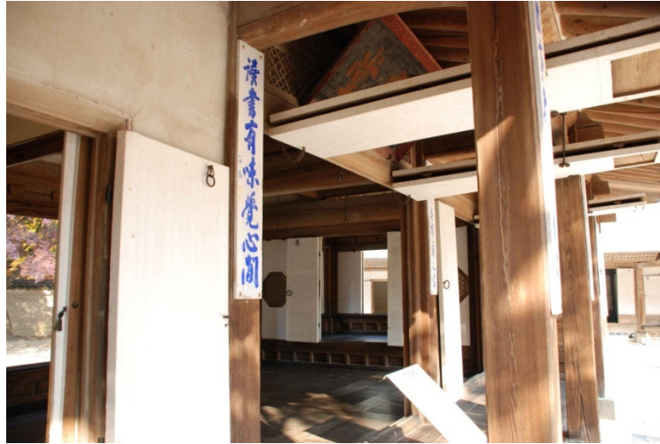
Figure 3-22 100% open possible oiled-paper windows in sarangbang , after opening the windows of half installed windows area, all windows hang over the ceiling or the roof eaves.
