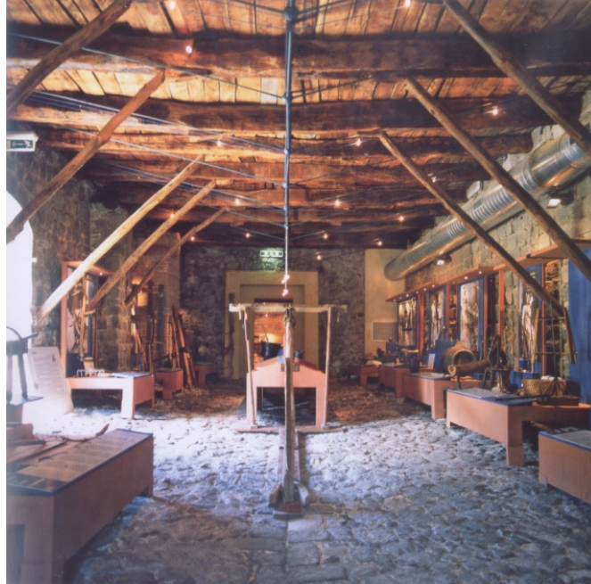
Figure 16. The exhibition hall, at the Museo della terra in Latera, Italy, reuses the traditional wood ceiling in a medieval barn. The ceiling is braced by modern metal tie rods. Because of their thin profile, the rods serve to disappear and become obtrusive. Source: Old Buildings Looking for New Use by Pierre Thiebaut, pg 191.
