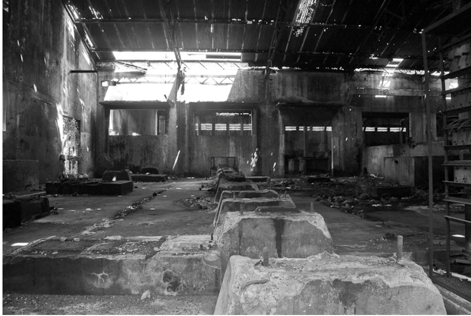
Figure 45. An interior shot of the manufacturing building. Here, a conveyor belt was once laid on the concrete pedestals. Source: http://www.mattprestonphotography.com/tag/travel/
