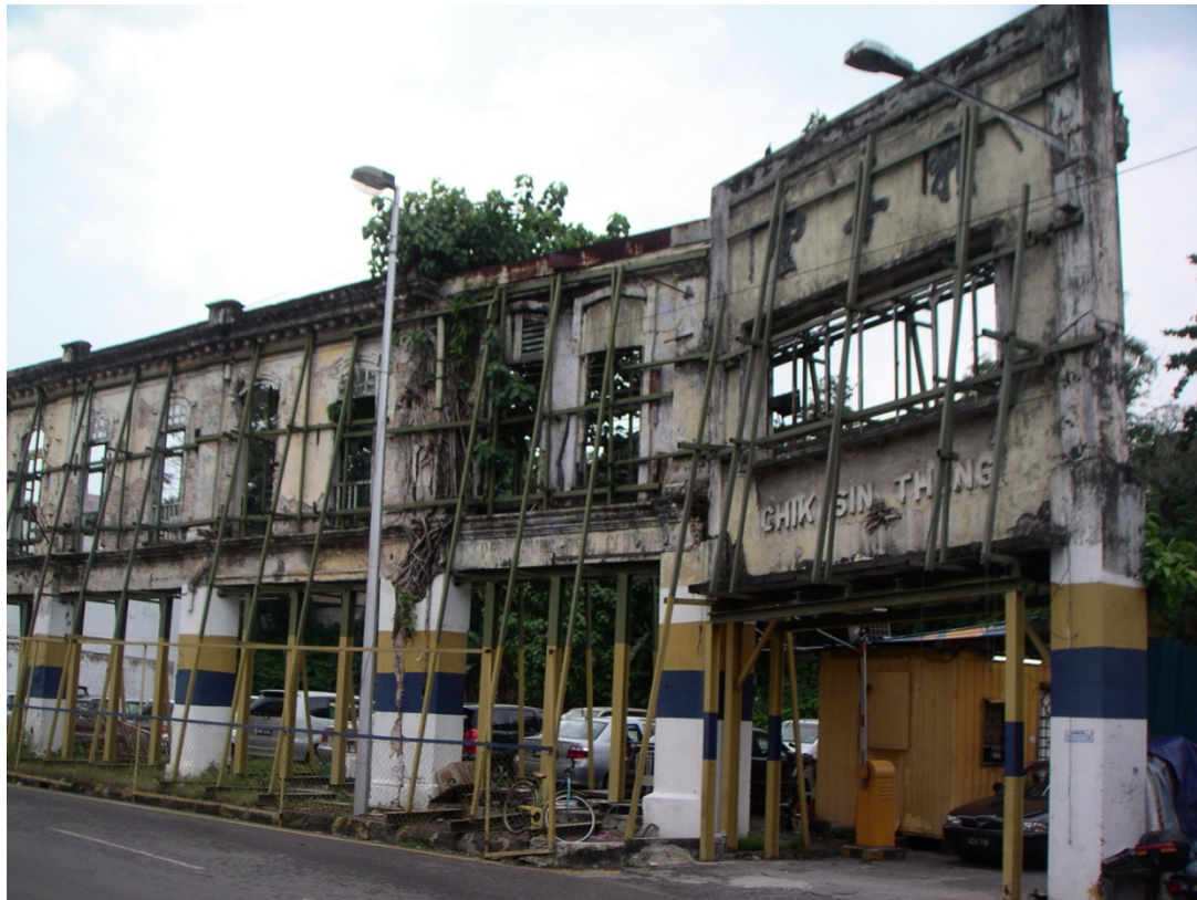
Figure 65. Heritage is often demolished without clearance of historical assessment. Here, the façade of the Chik Sin Thong Crematorium in Kuala Lumpur, Malaysia, demonstrates last-second supporting beams that precariously save the façade from collapsing. Source: Author's, 2005.
