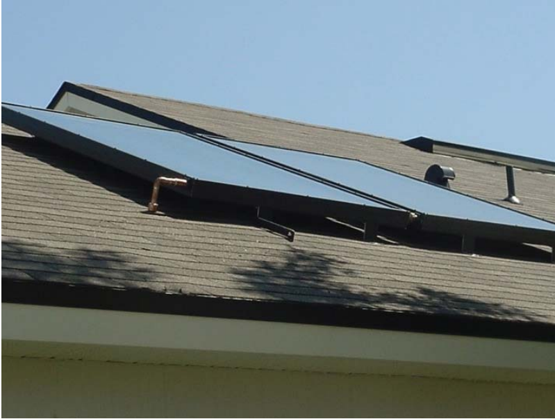
Solar Hot Water Heater collectors on a roof http://vikingsolarsolutions.com/images/solar_hot_water3_eiww.jpg
