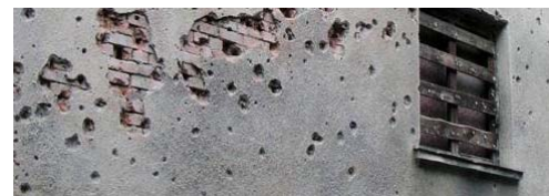
Figure 162. Bullet holes on a wall 385
