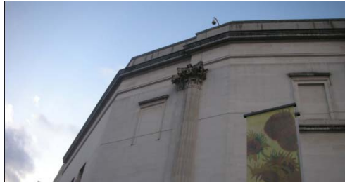
Figure 32. Façade illustrating window frames and sills, but no windows 192
