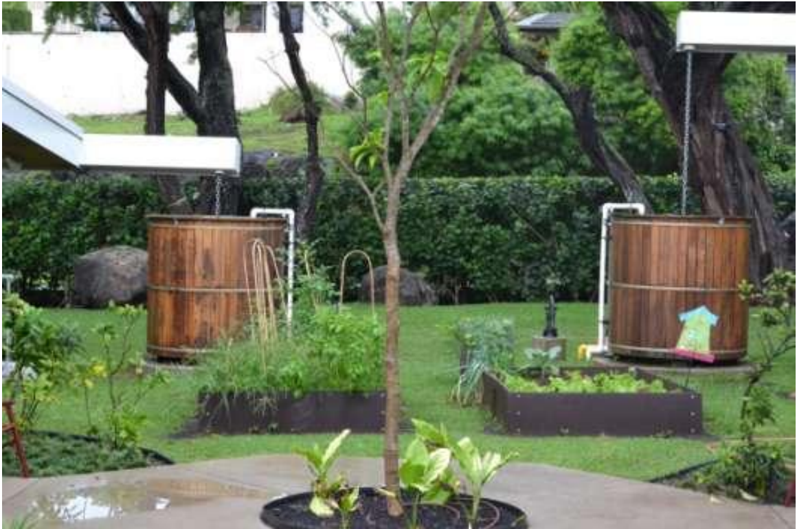
Figure 30 rain water catchment system near gardens
