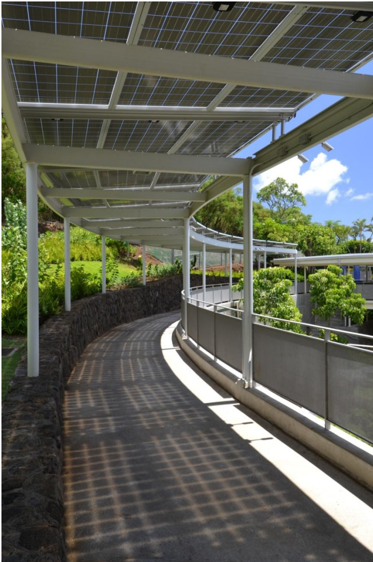
Figure 32 Photovoltaic panel roof on covered walkway 46
