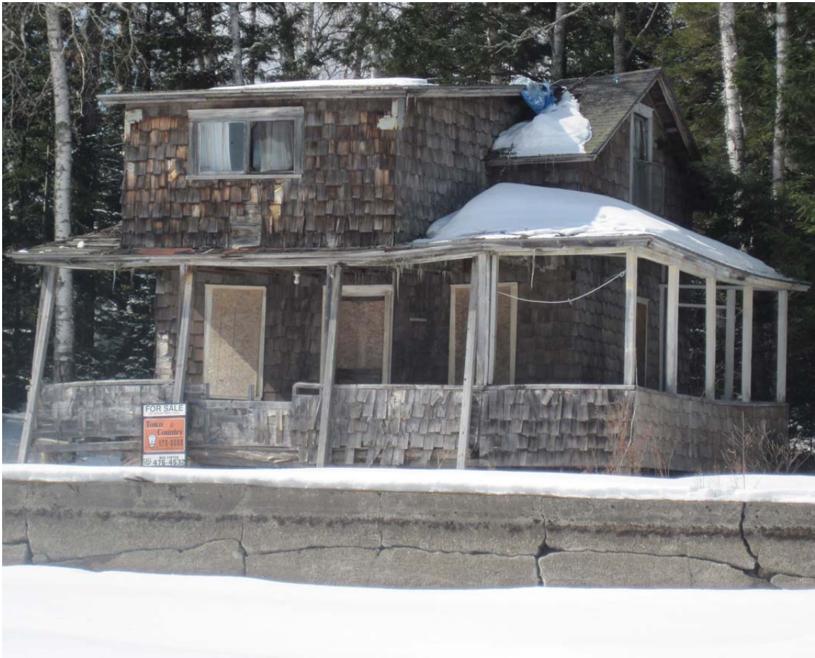
Figure 418. Existing Photograph - view of existing house condition from pond taken March 2012 by author
