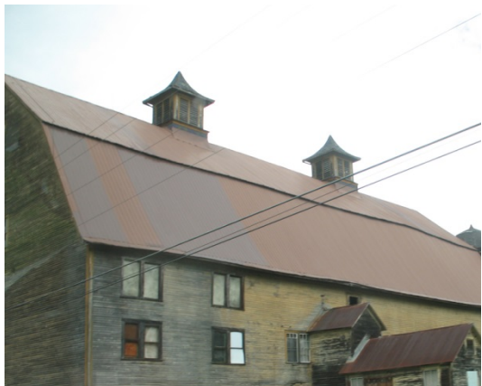
Figure 463. Site Context - view of large barn near Peacham in July 2012 by author
