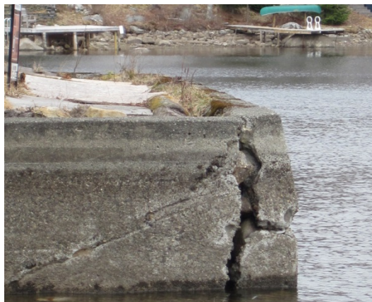
Figure 438. Existing Photograph - detail of sea wall failure taken in March 2012 by author
