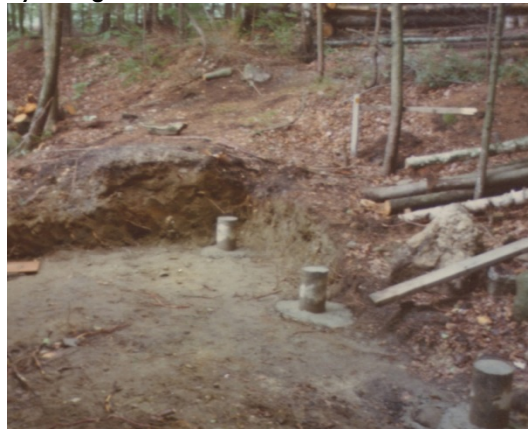
Figure 417. Historic Photograph - view of excavation for addition showing soil composition taken in the late 1970's by George Hudson
