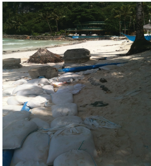
Exposed palm tree roots, sewage pipes, water pipes due to erosion and over-development. Sandbags also line the beach to prevent further sand loss and protect the tourist establishments.
