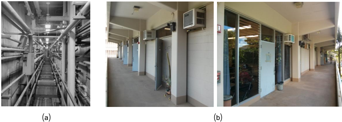
Figure 78: Laboratory Building of the HIG (a) Service shaft in the Laboratory building. (b) Window units placed into the louver windows.
