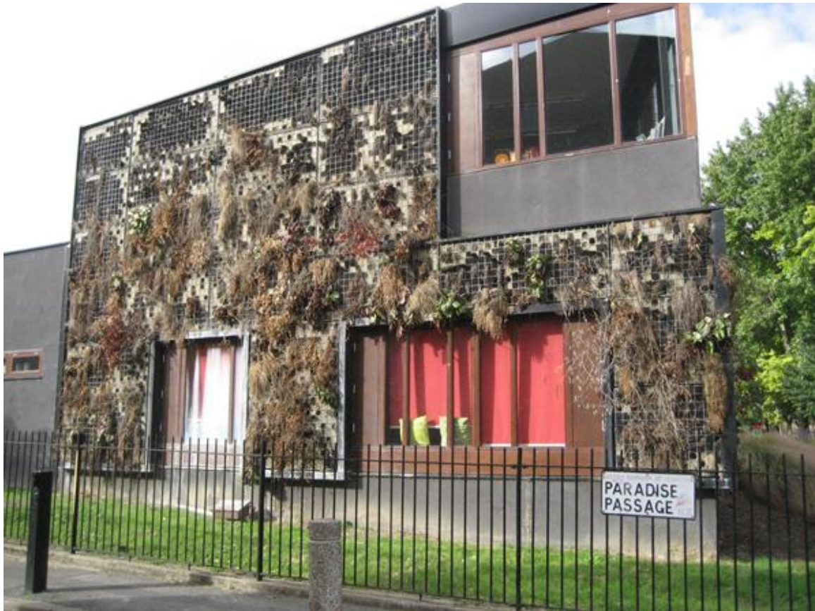
Figure 2.02 Failed Living Wall http://www.jetsongreen.com/images/old/6a00d8341c67ce53ef0120a5ac0b66970c-800wi.jpg
