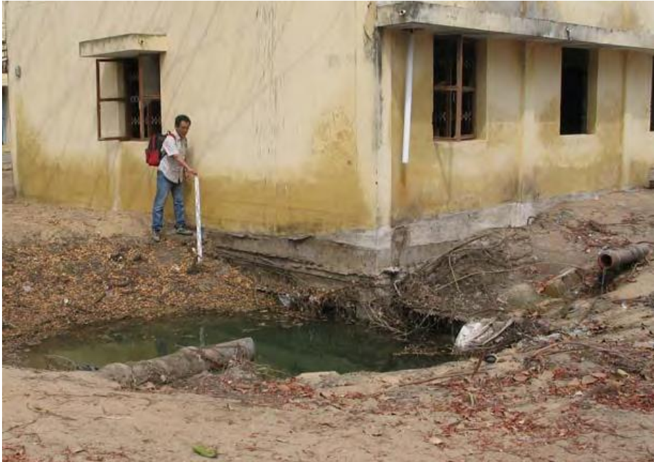
Figure 68: Failure of a sewage line due to scour Source: ORWARN 115
