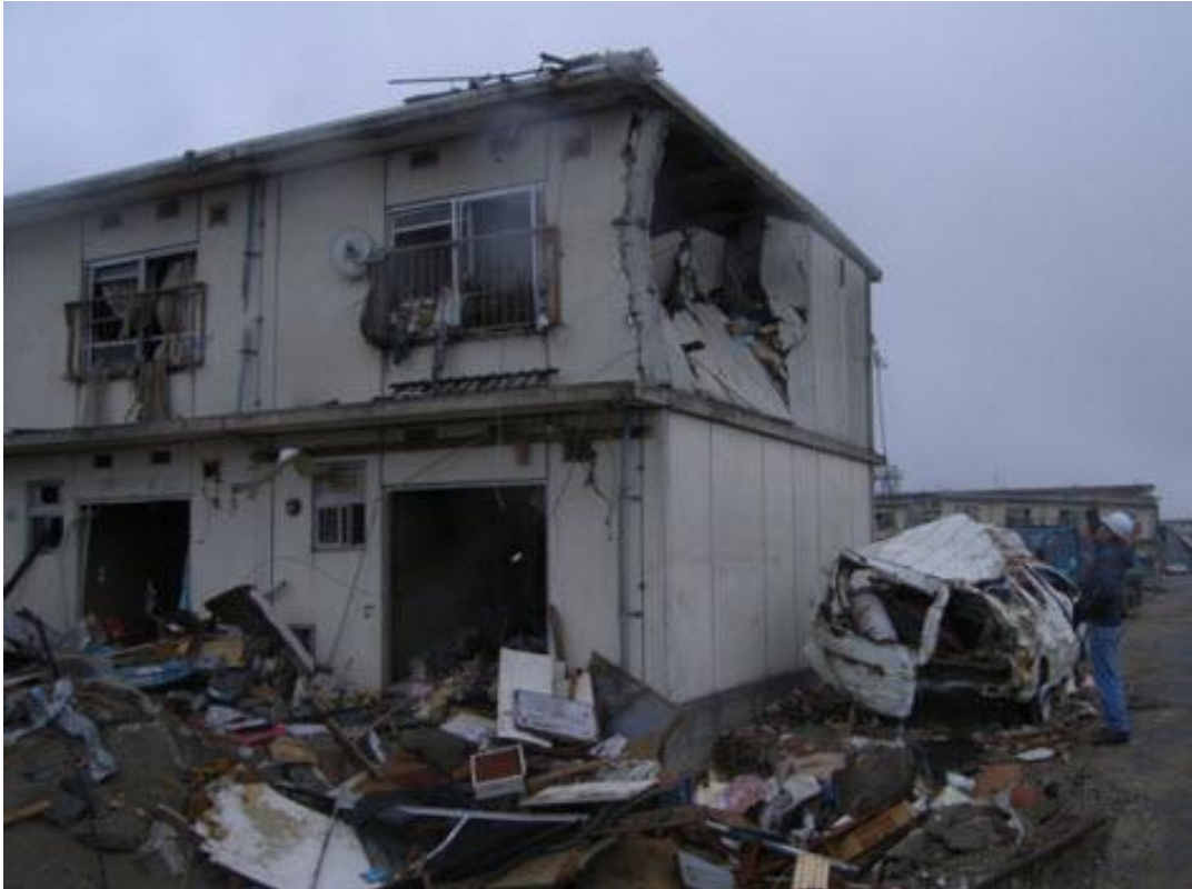
Figure 64: Debris impact damage in buildings, Natori Source: ASCE 2011 109
