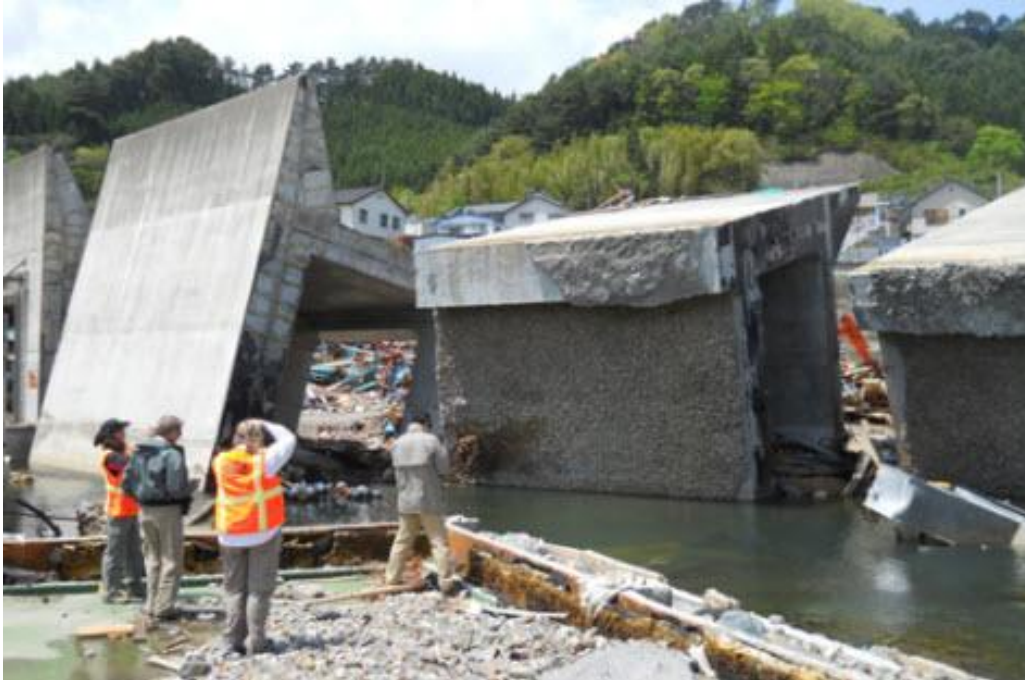
Figure 66: Overturned tsunami wall, Kohirahama. Source: ASCE 2011 112
