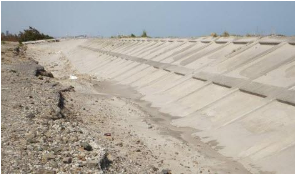
Figure 65: Scour in Sendai's Seawall Source: ASCE 2011 111
