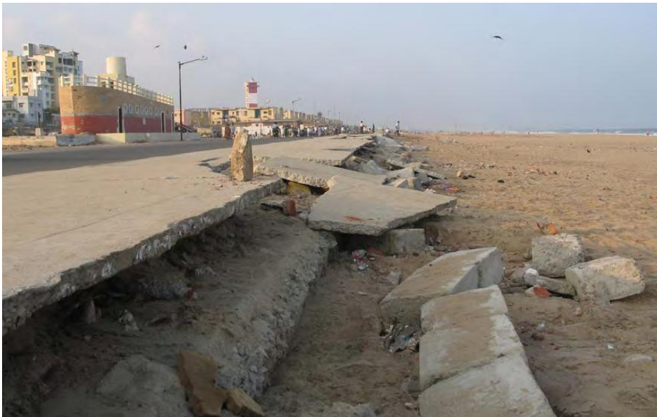
Figure 69: Collapsed concrete waterfront due to scour, Chennai Source: ORWARN 116
