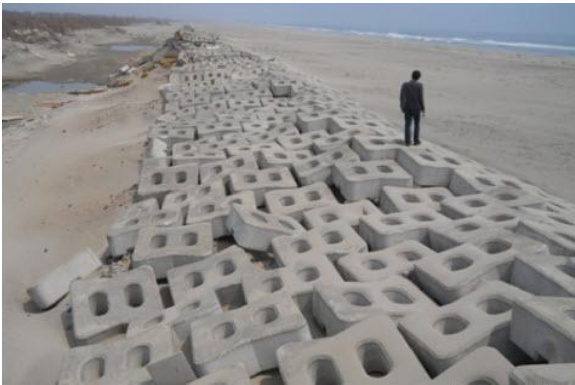
Figure 62: Failed section of Coastal Revetment Source: ASCE 2011 105
