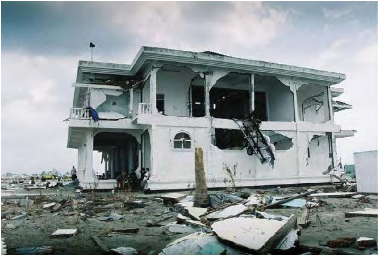
Figure 70: Concrete building after tsunami flood, Banda Aceh Source: ORWARN 117
