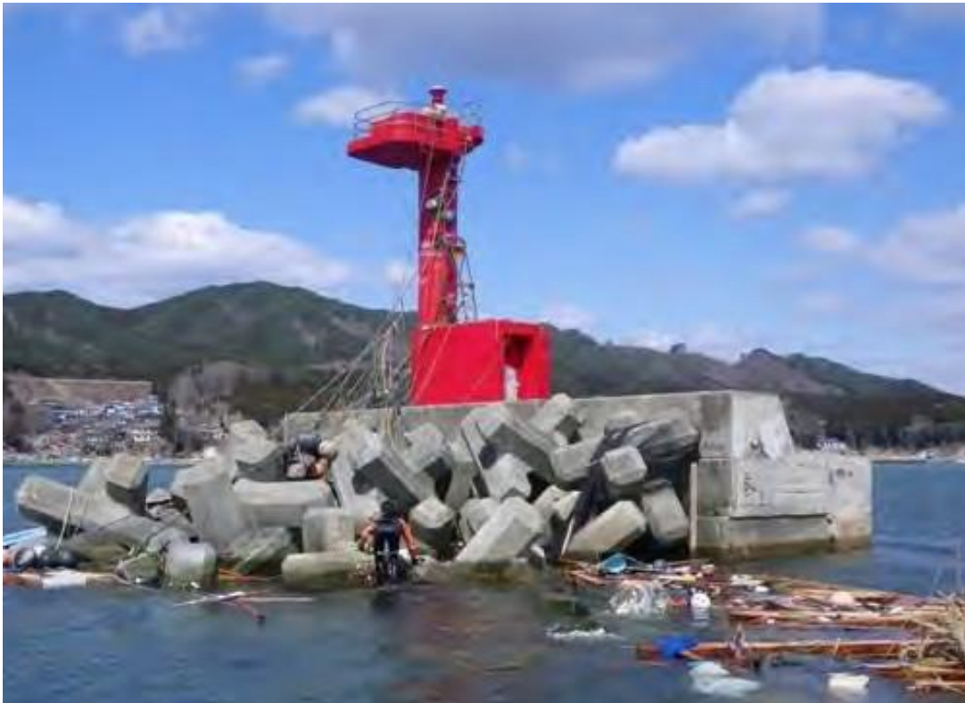
Figure 63: Collapsed Funakoshi East Breakwater Source: UNC 107
