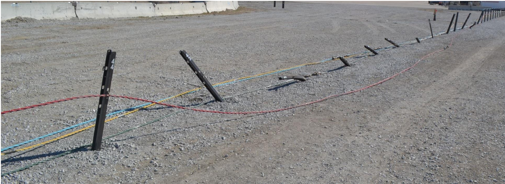
Figure 148. System Damage, Test No. MWP-7
