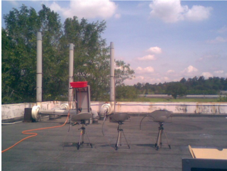
FIGURE 3. Solar dish concentrator setup systems in afternoon
