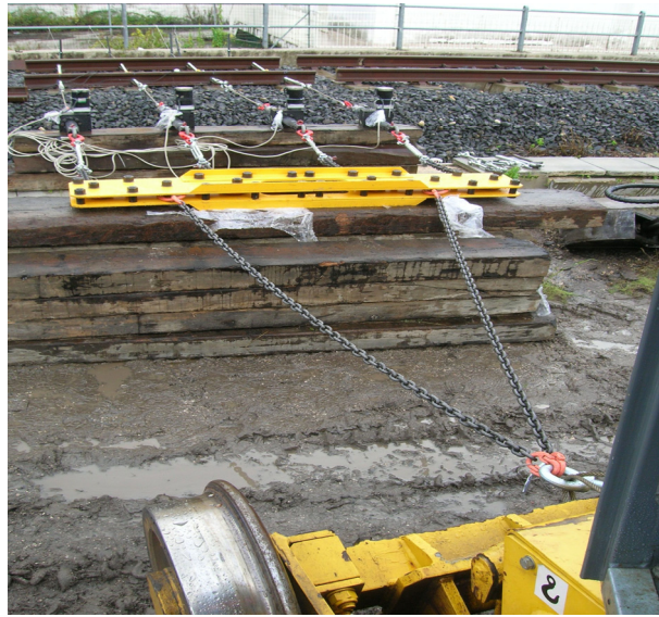
Figure 10b: Detail of the connection between the actuators and the fixed constraint.
