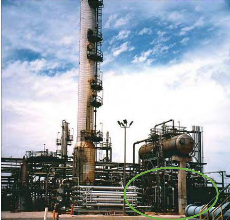
Figure 4: A skid-mounted membrane unit (circled in green) was installed to replace a bulky amine absorption process (in background)
