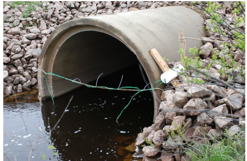
Downstream Antenna on Culvert
