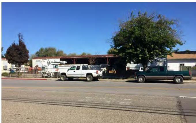
Figure 1.10: Paso Robles Street has fading paint through out the road.
