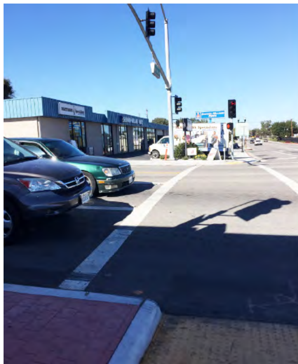
Figure 1.11: No pedestrian ramps on pedestrian crossings at busy intersections.
