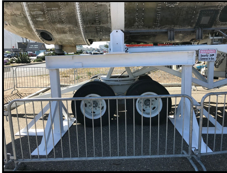
Figure 82. An image of the completed structure, as it will look when installed on the trailer.
