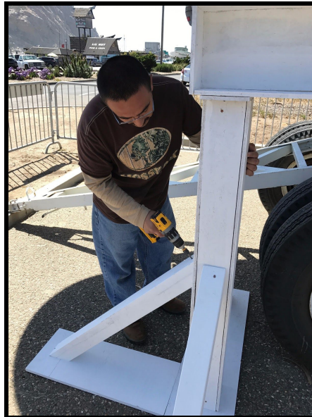
Figure 64. An image of Octavio connecting the short foot and strut to the column.
