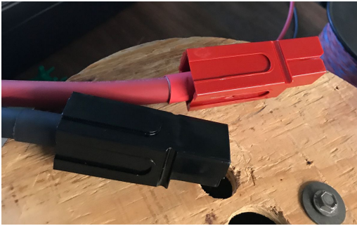
Figure 9: View of the Disconnect Cables
