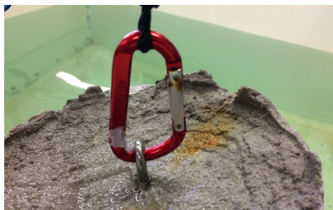
Figure 37: Corrosion found on the carabiner and concrete anchor during inspection.
