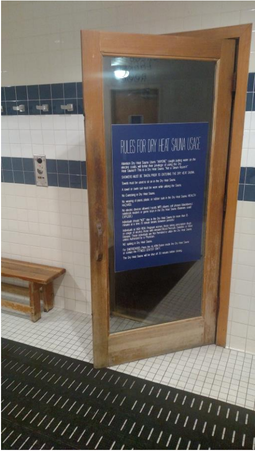
Figure 34 – Sauna Door Stuck on Non-Slip Floor Mat
