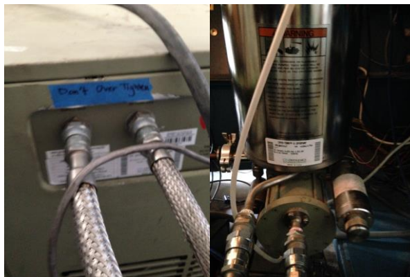
Left, compressor return and supply. Right, cryopump return and supply.
