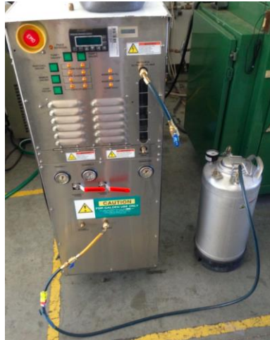
FILL LINES BETWEEN CHILLER AND PLATEN
