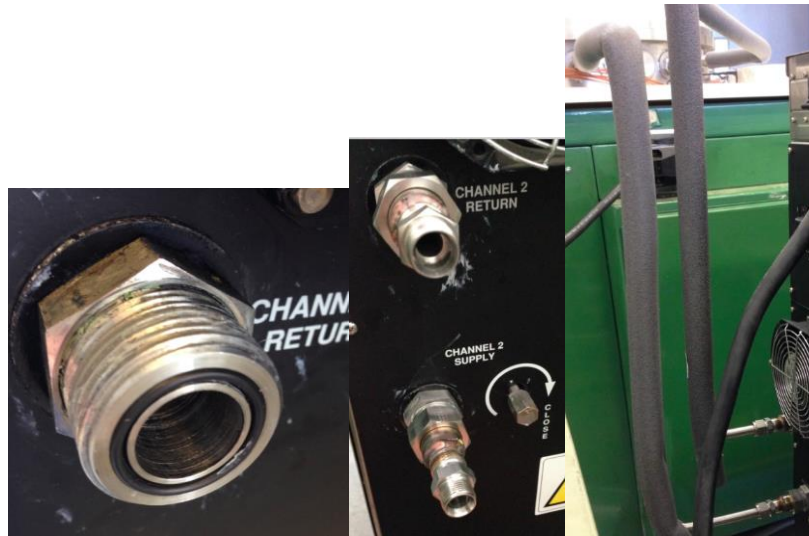
CONNECTIONS AT THE BACK OF THE ATS CHILLER
