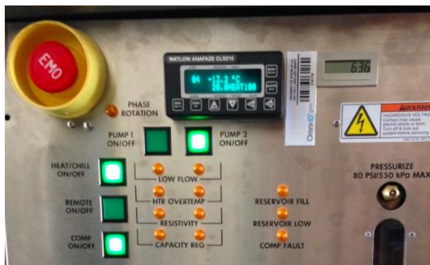
ATS CHILLER ON
