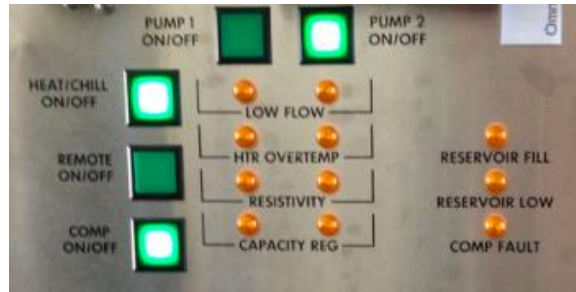
WARNING LIGHTS ALL OFF
