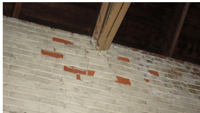
FIGURE 2 – POOL ROOM TRUSS CONNECTION
