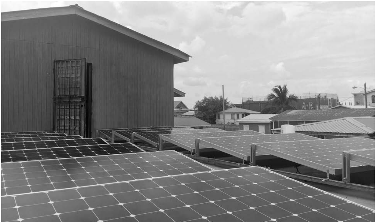
Figure 1: Solar panels installed for San Pedro Roman Catholic Primary School.
