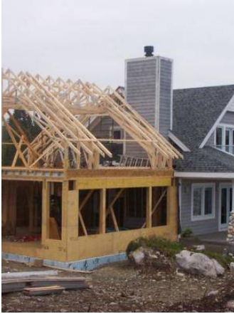
Any addition should be designed to look like part of the original house
