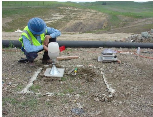
Figure 21 – Photograph of Sand Cone Test being Conducted within the Tested Chamber Perimeter
