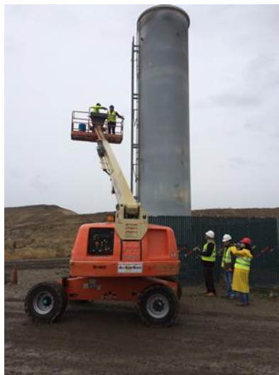
Figure 22 – Photograph of the Flare System and Boom Lift at PHL
