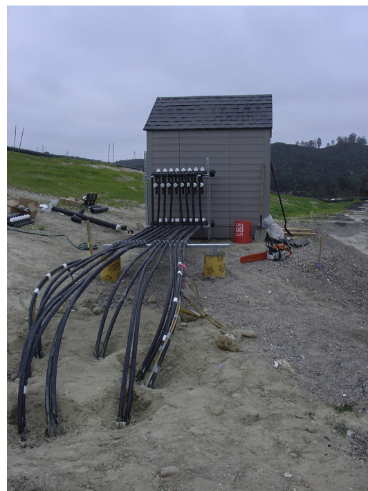
Fig. 6. Photograph of pilot heat management system.
