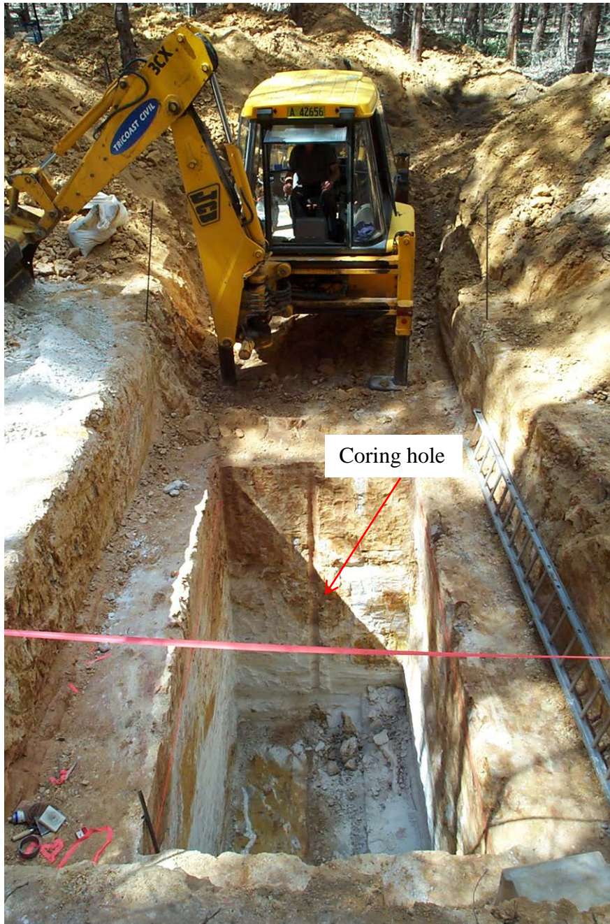
Figure 4.2 Excavation of the 7 year tree root system at an excavation depth of approximately 6 m, coring hole visible in the excavation pit wall.
