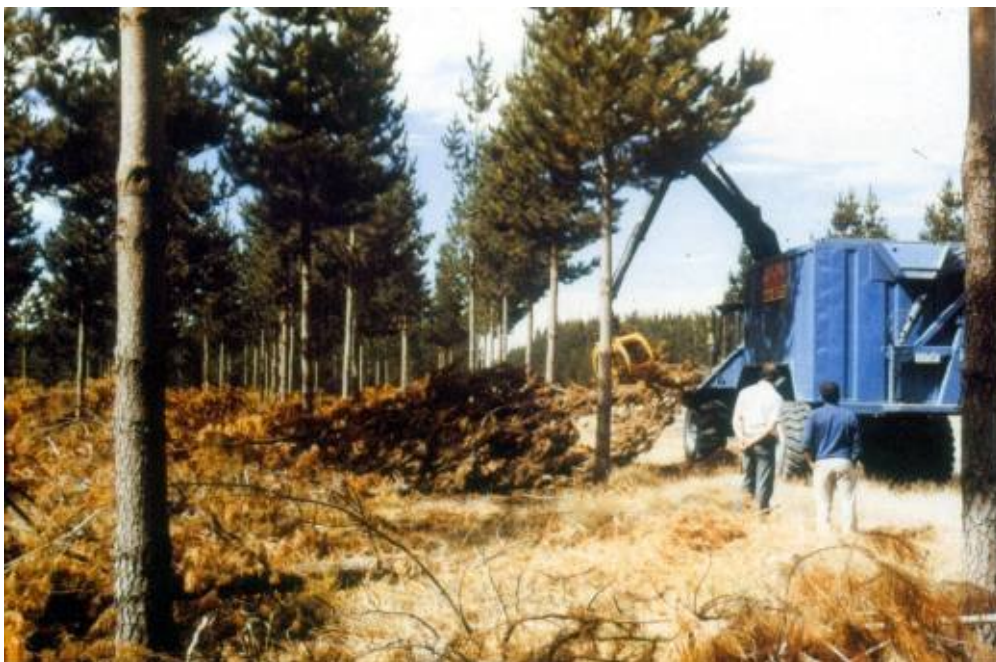
Figure 6-16 Using large mobile chipper to collect and chip P. radiata plantation thinnings
