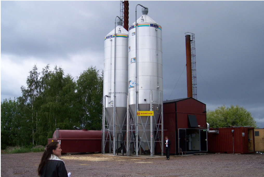
Figure 8-4 Wood pellet fuelled central heating plant in Sweden
