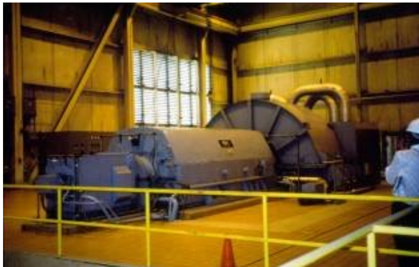
Figure 14-3 Steam turbine driving a 25 MW e generator in a wood-fired power plant in Canada
