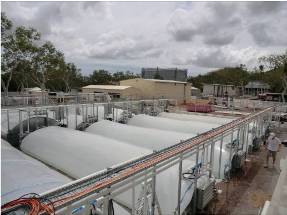
Figure 20-10 MBD R&D Facility at James Cook University, Townsville, Qld
