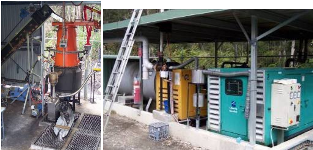
Figure 13-14 Ankur gasifier in Huon Valley, Tasmania and dual-fired diesel generator set
