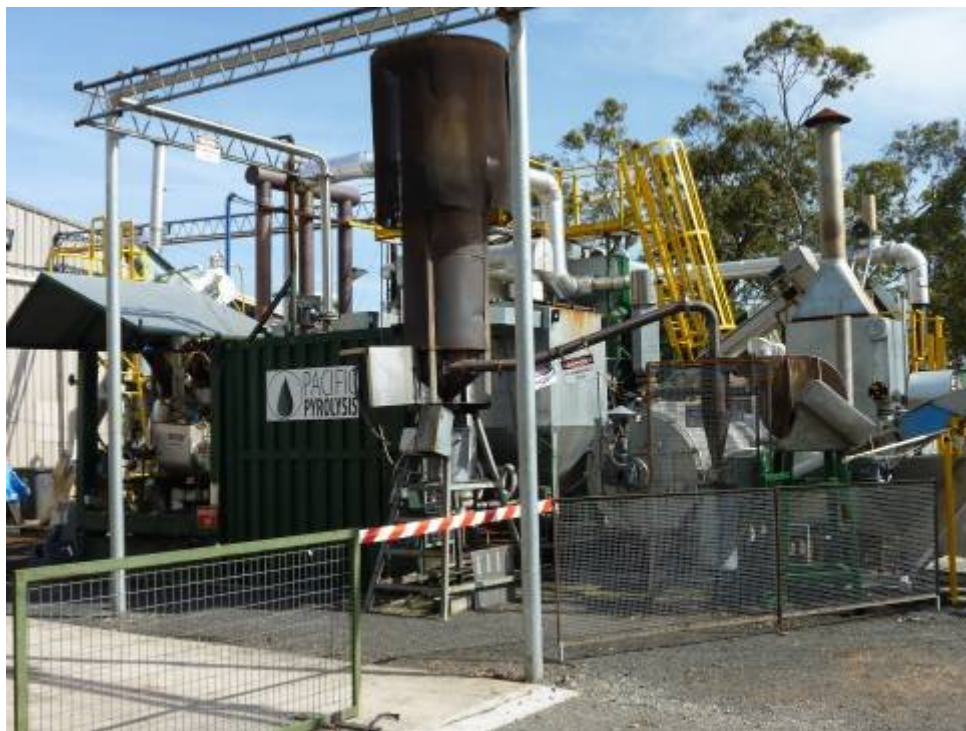
Figure 13-18 Pacific Pyrolysis demonstration plant, Somersby, NSW
