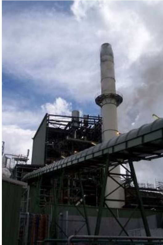
Figure 13-5 30 M cogeneration plant at Condong Sugar Mill
