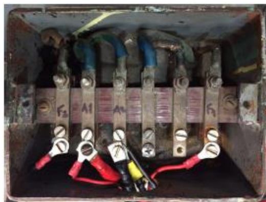
Figure 13: Wiring in the terminal of generator [14]
