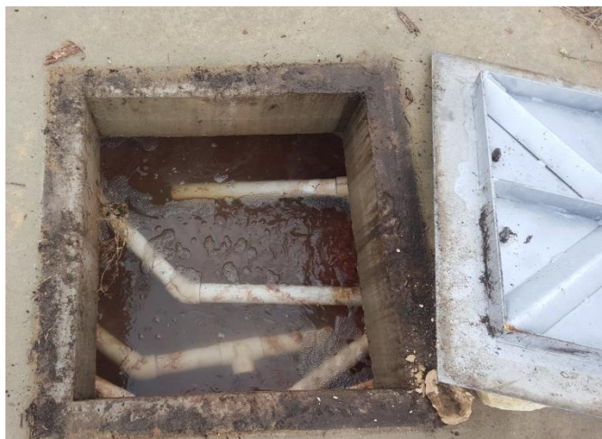
Figure 5. Picture looking into one of the Envirophos Tanks at Timbers Edge, taken on the 26/04/16
