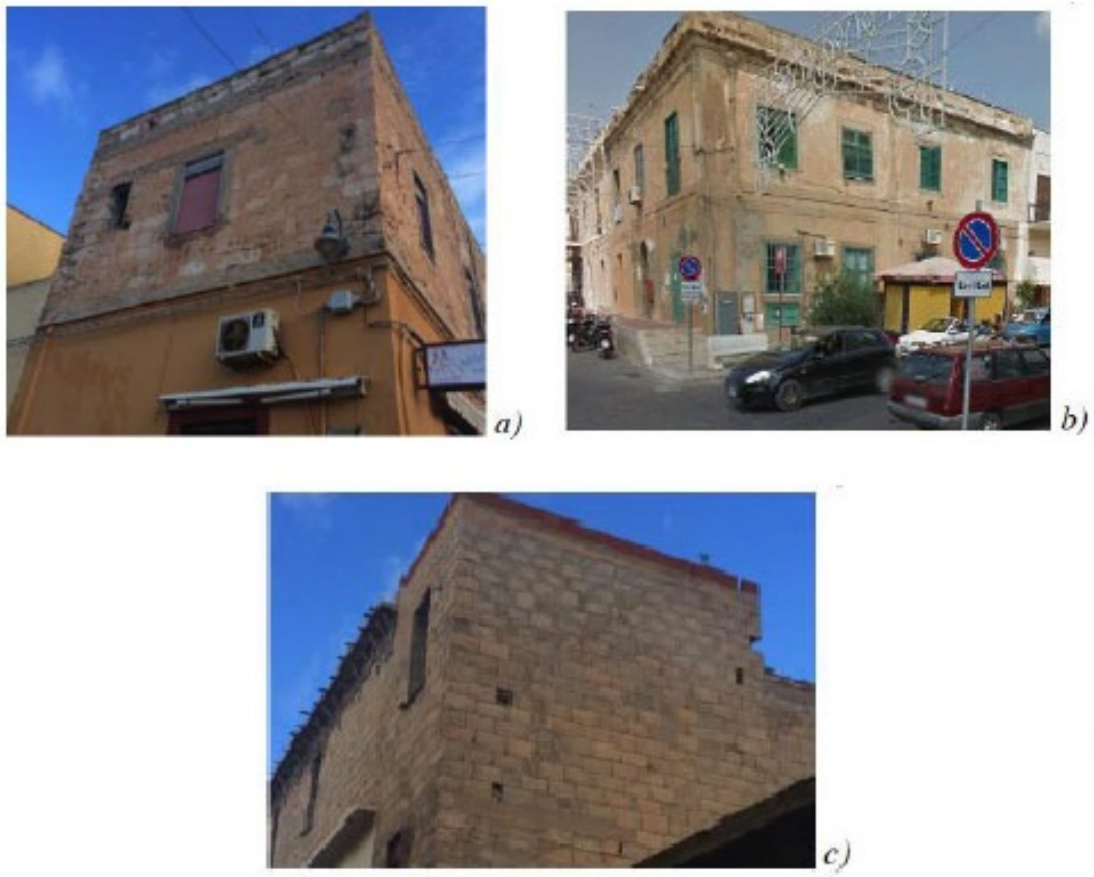
Fig. (4). Typical masonry buildings in the urban centre of Lampedusa: (a, b) Calcarenite masonry; c) Concrete blocks masonry.
